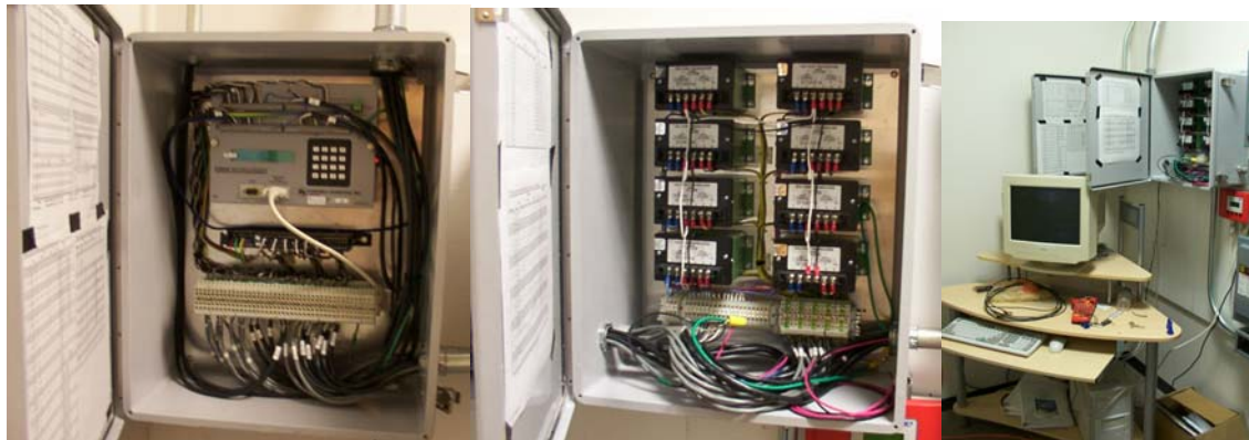
Figure 22 Data Logger Box, Transducer Box, and Overall Setup
