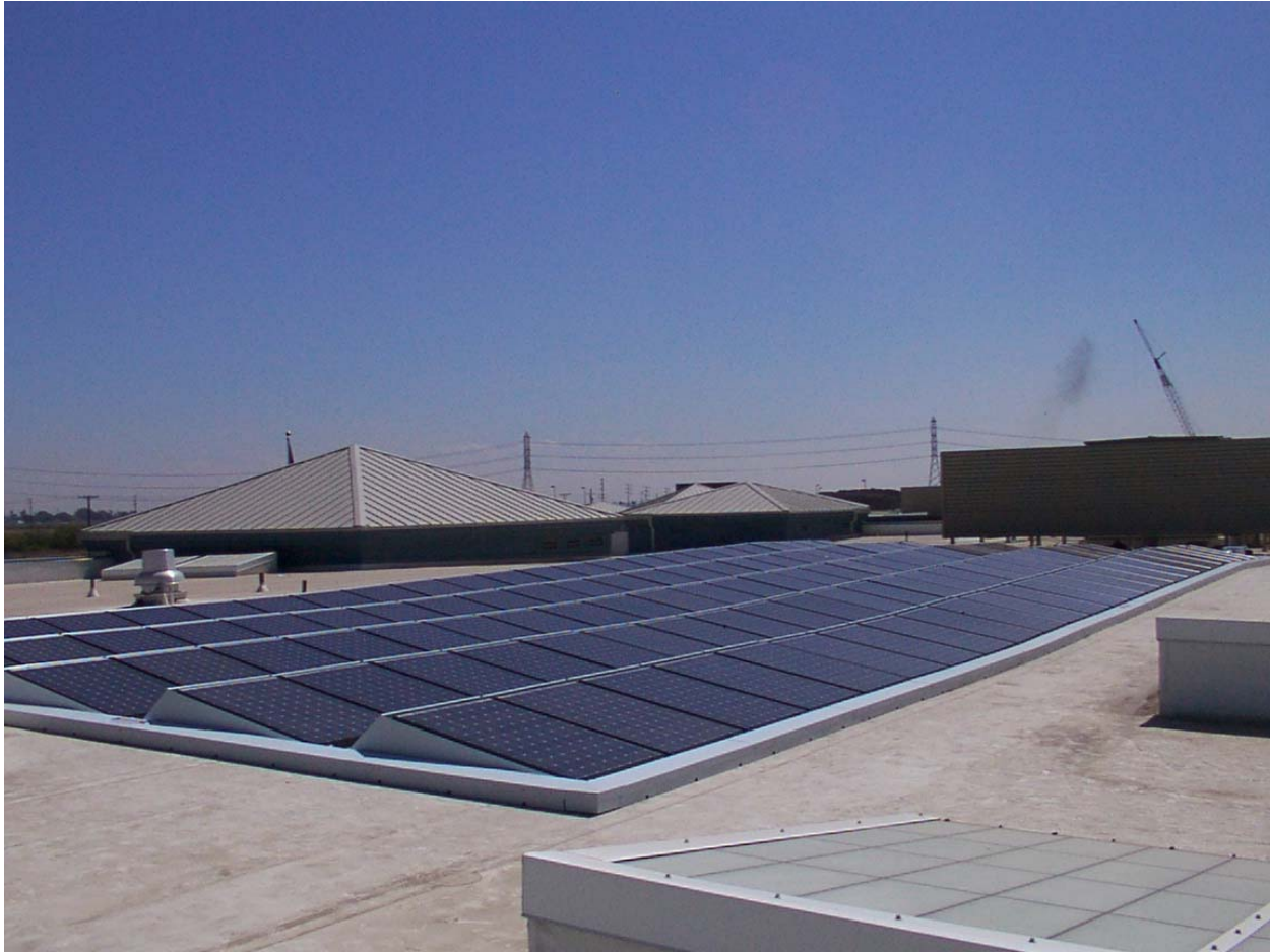
Figure 1 PowerLight Sloped PowerGuard 20kW PV System
