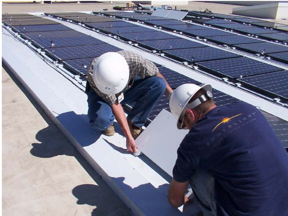
Figure 13 Lifting module-shroud assembly and snapping shroud into slots (home run wire for series strings already in place)
